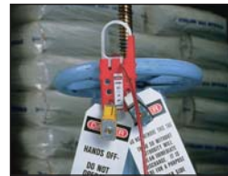
Lockout gate valves
